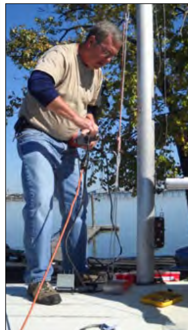
Dick using a drill to remove the rivets from the old broken mast ring to which the spinnaker pole secures. Photo by Chris Von Guggenberg.
