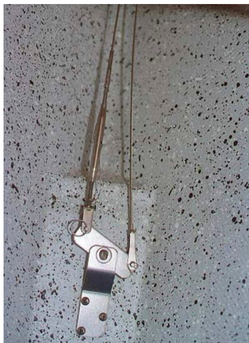
THIS IS A CLEAR PICTURE OF HOW THE TOGGLE PLATE SHOULD LOOK. IT PIVOTS AROUND A RIVET ATTACHED TO THE LOWER BRACKET. THIS RIVET IS WHAT FAILED. PHOTO CREDIT: ERIC SCHMIDT
